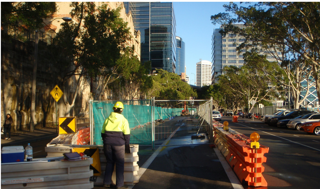
July 2011: Laying high voltage cables in Hickson Road to power the Barangaroo South site
